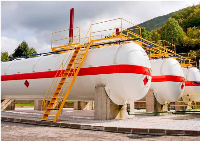
Natural Gas Containers
